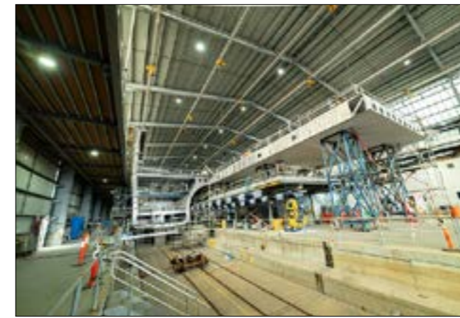
The Buquebus stern under construction at Incat Tasmania Photos © Incat Tasmania Pty Ltd
