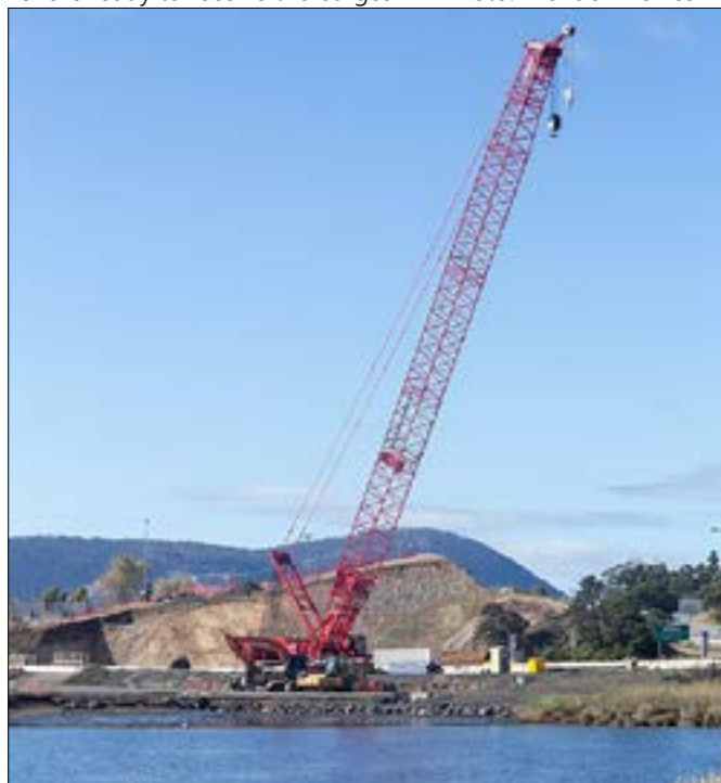
below: Ground works and reclamation underway on western shore ready to receive the barges Photo: Brendon Bowes
